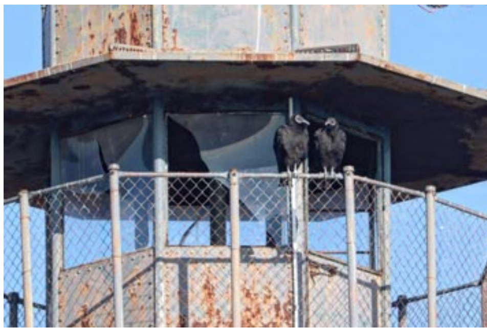
Mattamuskeet Lodge and observation tower, considered a state treasure, recently was leased to Hyde County for restoration and $6.5M allocated for initial repairs by the legislature.
